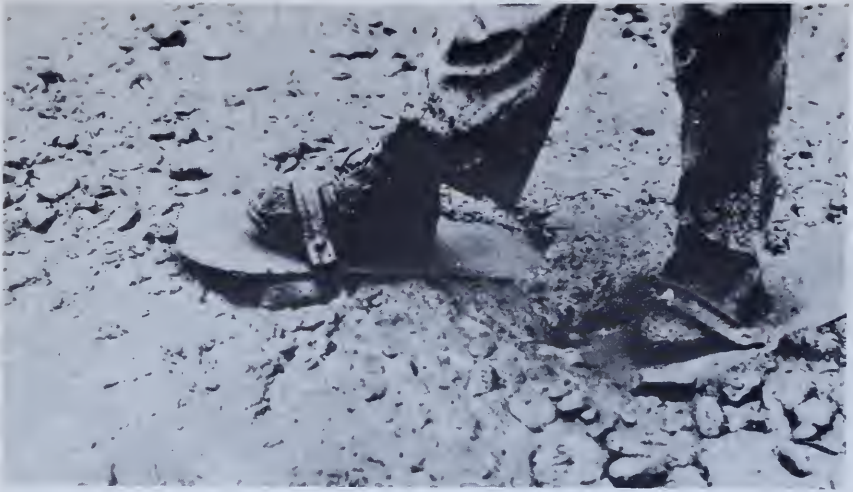
Figure 120.—Workman wearing “snowshoes” on a fresh joint surface. Snowshoes minimize undesirable working of the concrete and facilitate cleaning of the surface. PX-D-33053.
